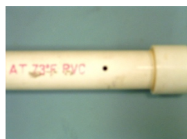
1. Pipe with pin hole. Relieve pressure. Surface can be wet or dry.
