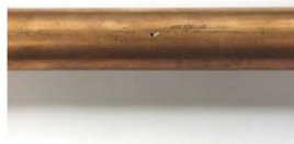
1. Pipe with pin hole. Relieve pressure. Surface can be wet or dry.
