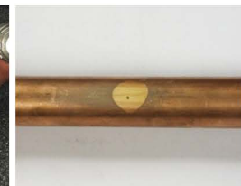
6. Remove NSR Tab. Completed repair. Note resin covers an area larger than the actual hole.
