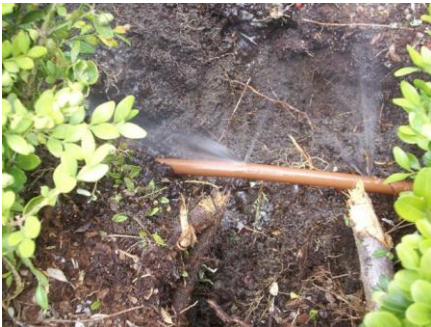
Pic 1. Holes caused by landscaping company
